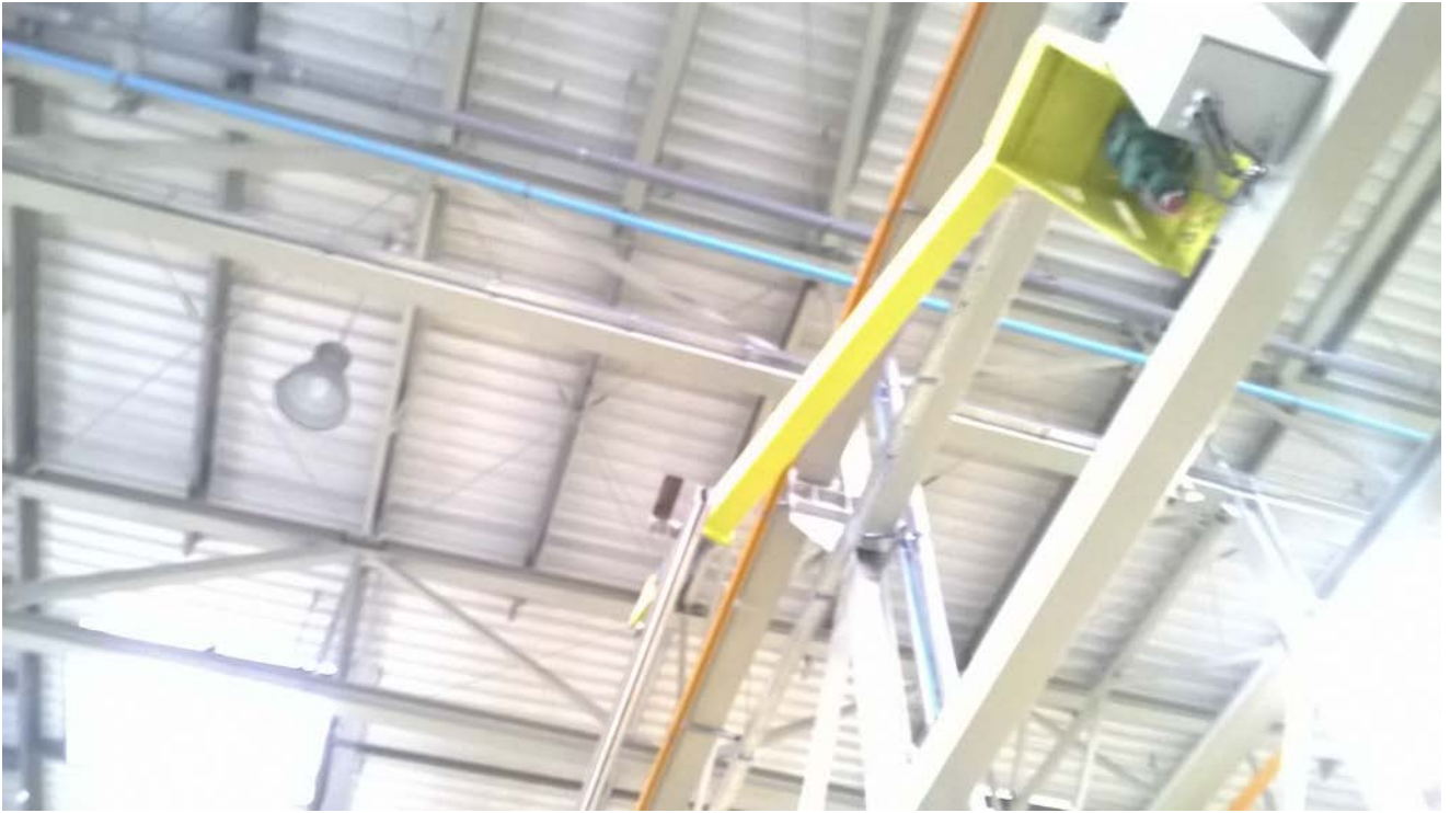
Photo 8: Movable rigid catenary with a motorised arm in the Alstom Workshop
